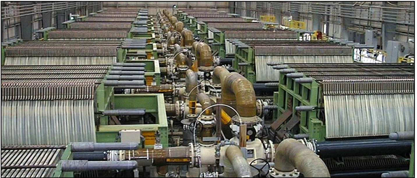
Covestro, Baytown – Chlor-Alkali Cell Room (Image Courtesy of Covestro LLC)
